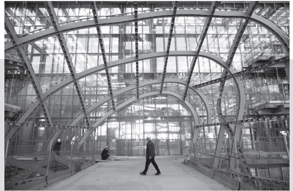
An interior view of the construction of a new meeting centre 'La nuvola' (The cloud) in Rome, Italy, 25 November 2013. The building by Italian architect Massimiliano Fuksas will be inaugurated in 2015.
